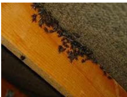
Cluster Flies in loft area
